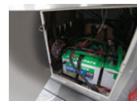
BATTERY TRAYS AND BREAKERS UNDER CENTER CONSOLE W/TOE KICK
